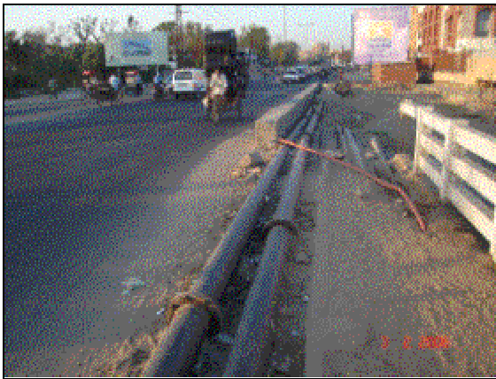
Water supply pipelines along road
